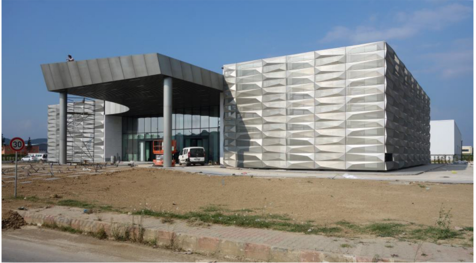
Fig. 8. Front of Sakarya Industrial Zone Headquarters and Conference Hall , Sakarya, Turkey, under construction, completion September 2016. Photo credit: BINAA.
